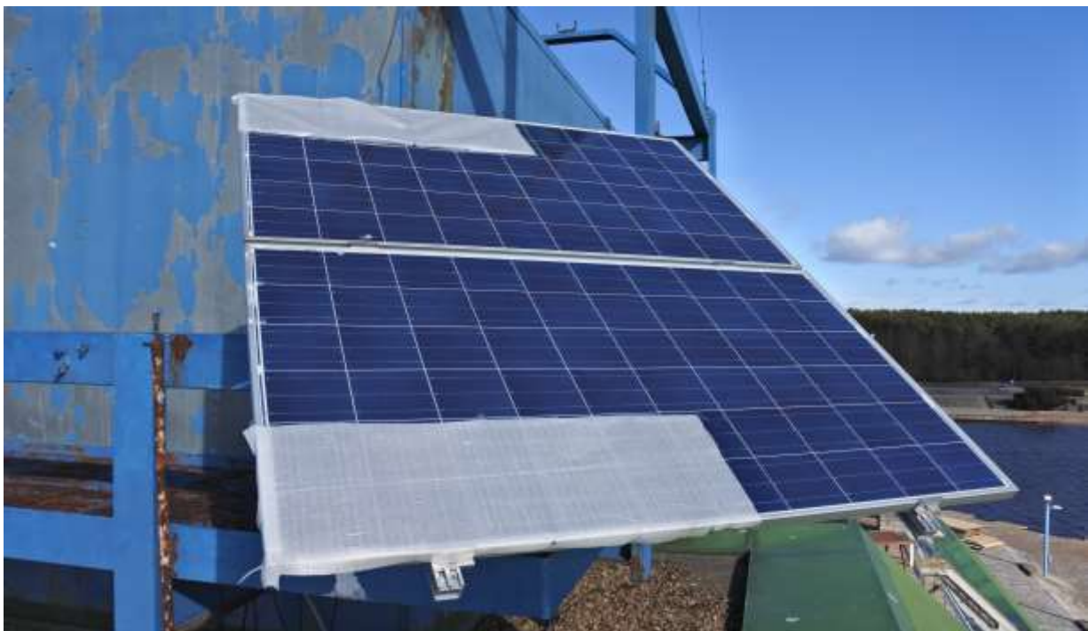
Fig. 3. Pirita 1 permanent grid-tied installation with two Naps Saana 250 SP3 MAW PV modules (2x1 substring shaded)
