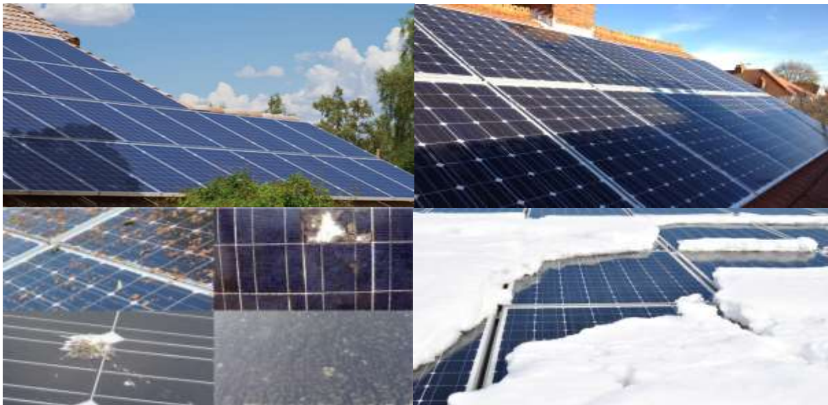
Fig. 1. Conditions resulting in partial shading of the residential PV installations
